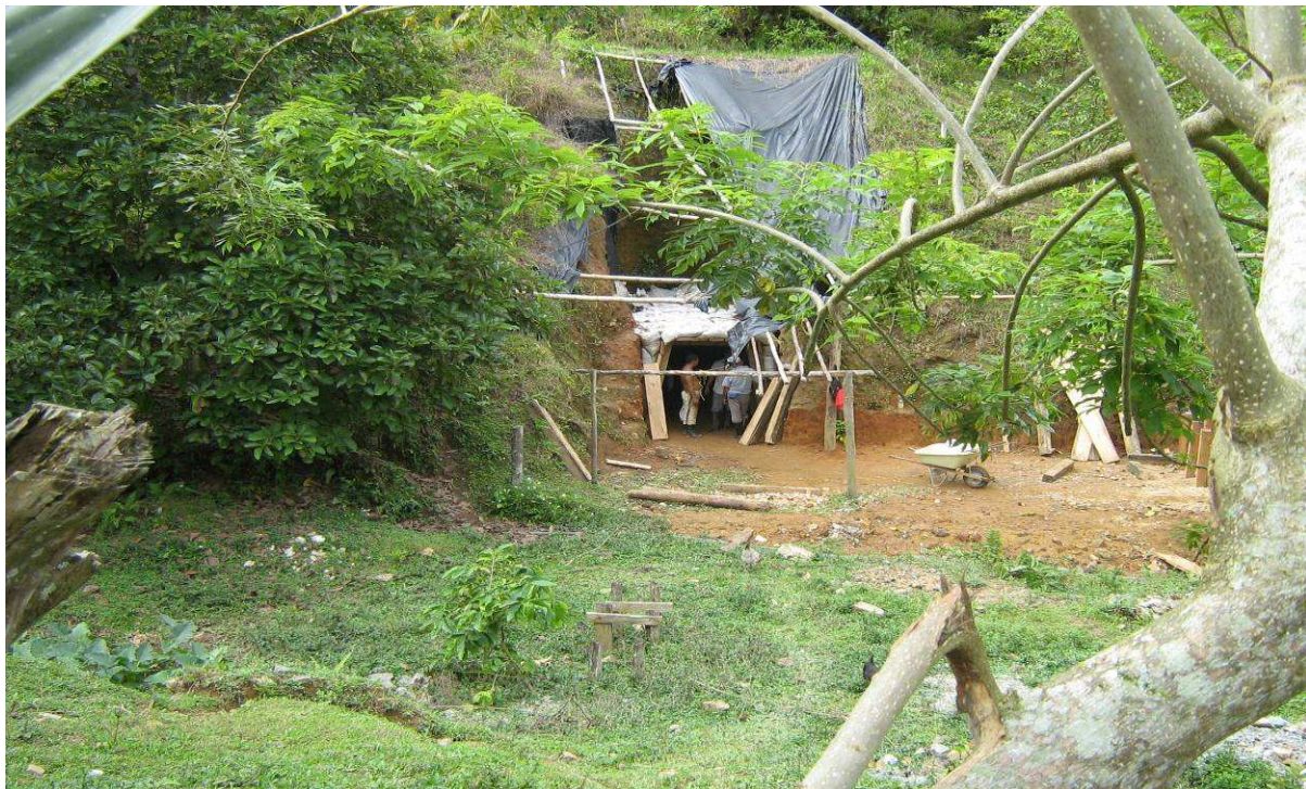
THE FIRST TUNNEL ROOF AND OFFICE HAVE NOT BEEN BUILT YET. THE TEAM AT THE MINE IN SEGOVIA COLOMBIA HAS MADE TREMENDOUS PROGRESS SINCE NEW MANAGEMENT TOOK OVER IN OCTOBER 2009!
