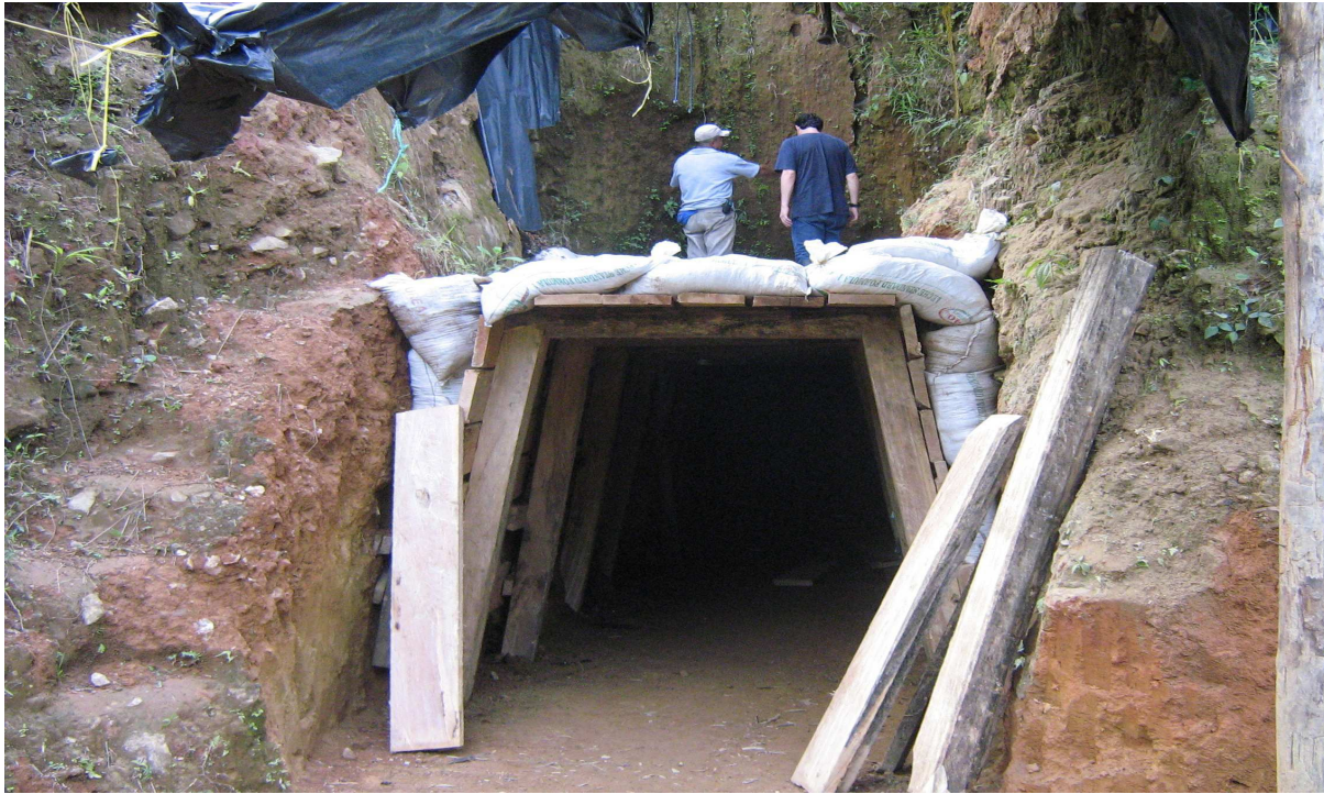
APRIL 2009 MINE # 4395 LAS PALMERAS AS THE FIRST HORIZONTAL TUNNEL WAS BEING REBUILT FROM SCRATCH!
