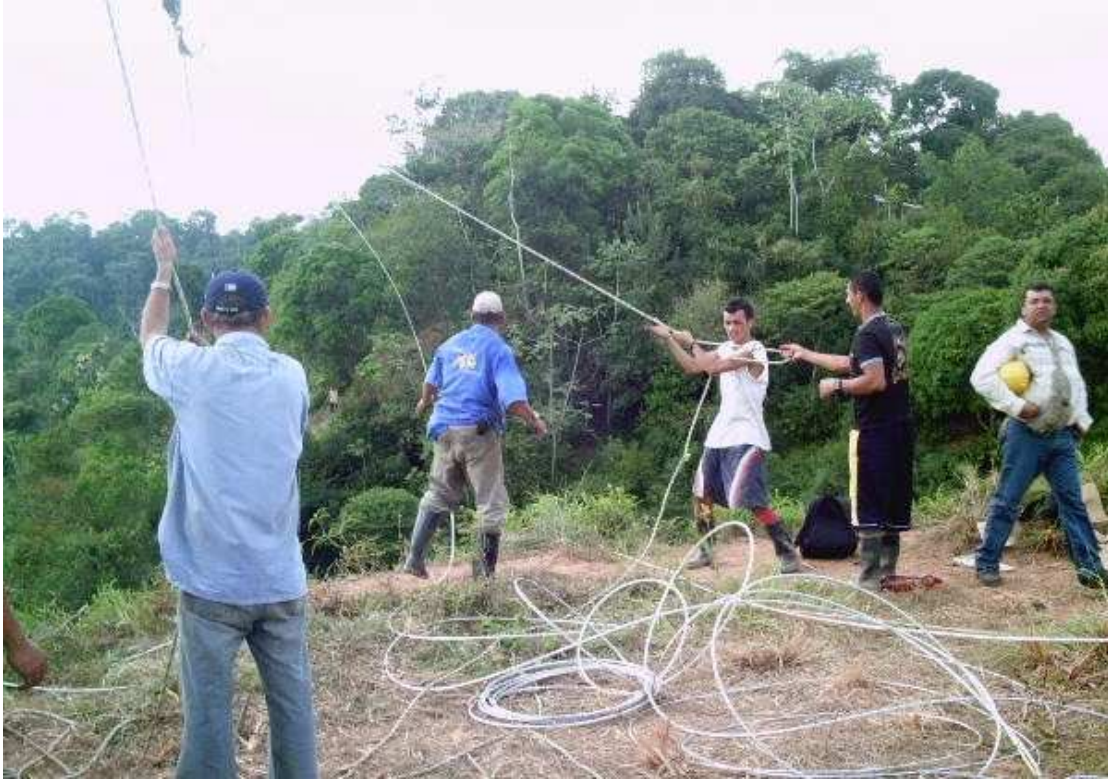
LABORERS LIFTING UPRIGHT THE 10 METER POLES AFTER CARRYING THE EQUIPMENT 600 TO 700 METERS INTO THE HILLS ON THEIR SHOULDERS.
