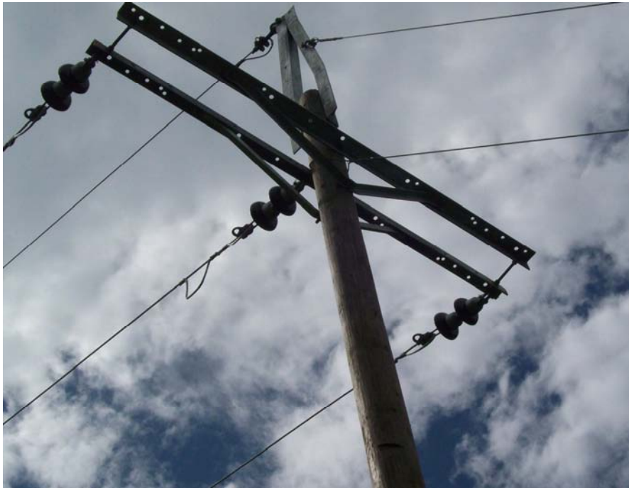
THE FINAL PRODUCT: A HIGH INTENSTIY LINE THAT CAN PROVIDE ELECTRICITY FOR A MINE AND PROCESSING PLANT.
