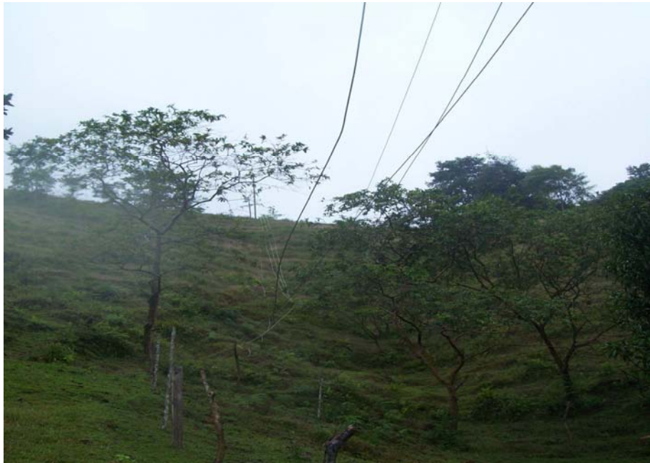
HIGH VOLTAGE LINES RUNNING DOWN THE HILL TO THE MINE ENTRANCE
